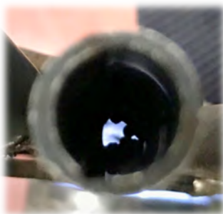
NH3 KNIFE FOUND TO BE PARTIALLY PLUGGED.
